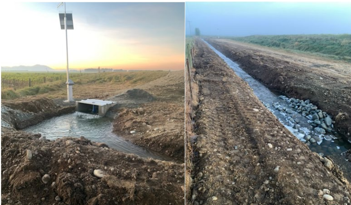
Figure 3-5: New MAR08 flow control device and connection to recharge race (Source: HHWET)
