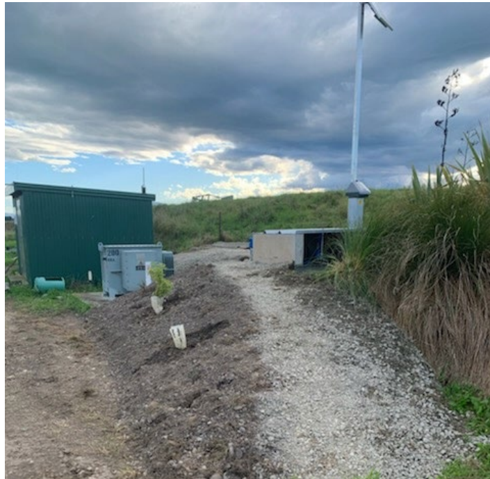
Figure 3-4: New MAR16 flow control device and connection to recharge area (Source: HHWET)
