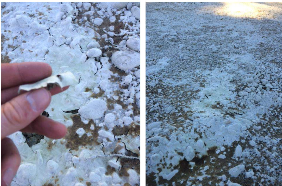
Figure I6: MAR basin clogging layer as seen in infiltration basin.
