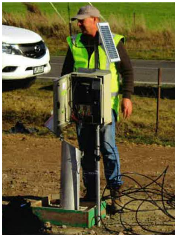
Figure 2: Bore head of GWD-01 monitoring bore: showing cable for sensor and power supply enclosure.
