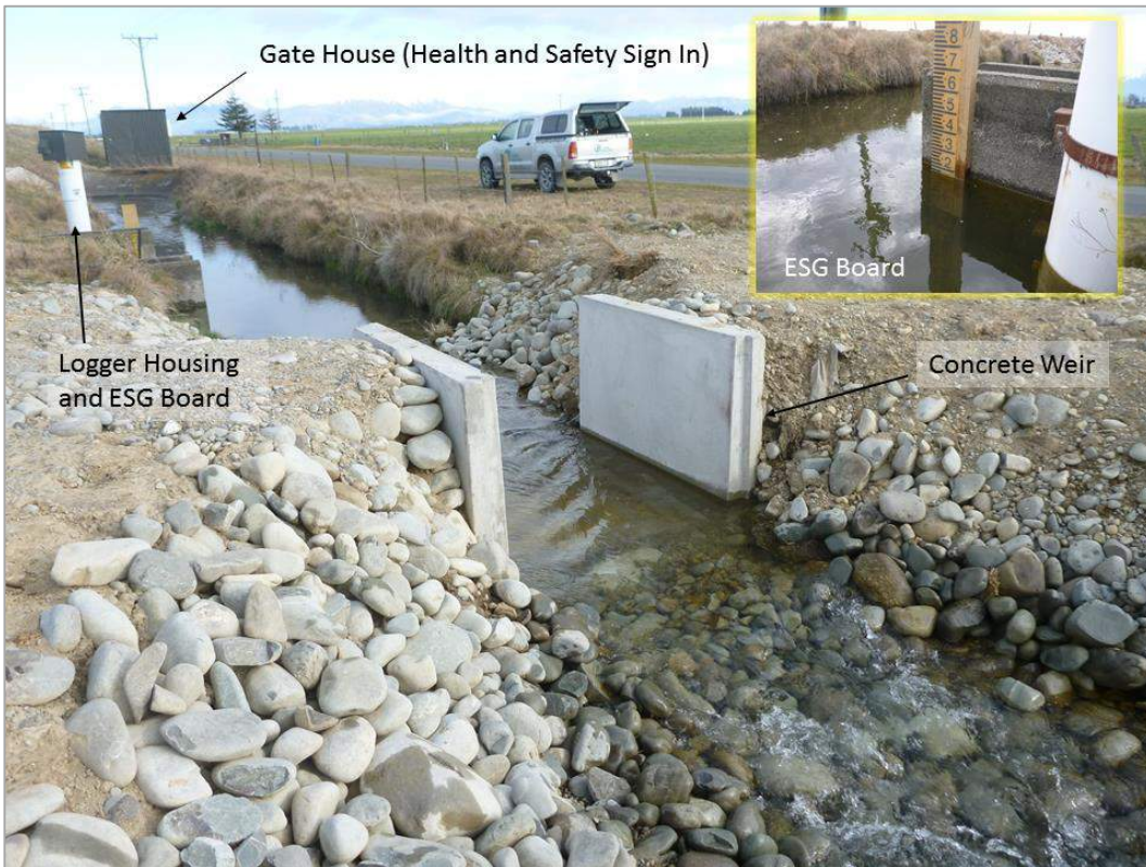
Figure E5: Flume 1 with Valetta Pond #3 gatehouse, ESG board (inset) and logger housing.
