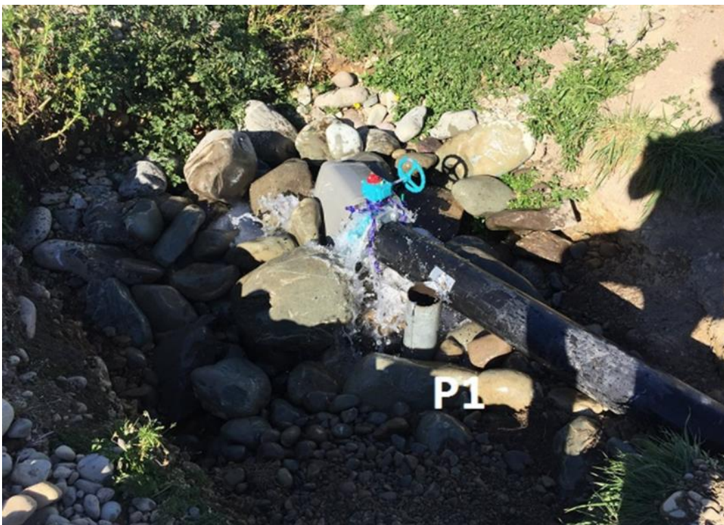
Figure F28: MAR13 site flow control system.
