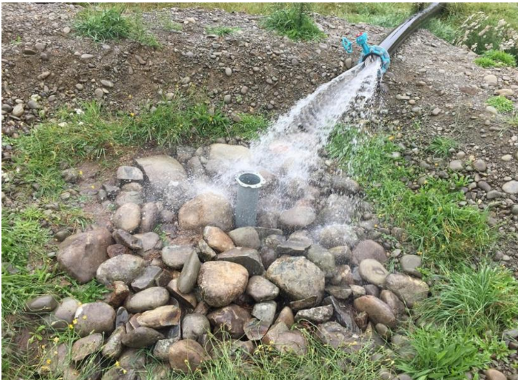
Figure F16: MAR08 site flow control system.
