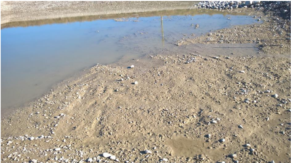
Figure 17: Sediment clogging in settling basin (forebay) following Year 2 scheme shutdown (July 2018).
